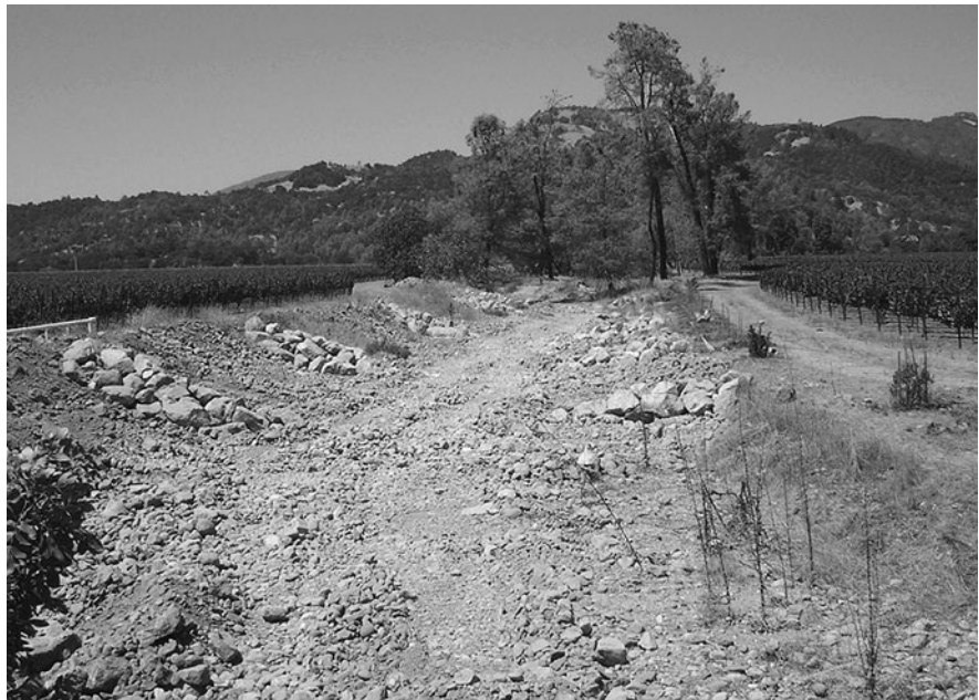
Fig. 3 Habitat restoration project on Selby Creek, Napa Valley, California. Over 100 boulder structures were installed in the channel of Selby Creek with the intention of inducing bed scour and creating pools for fish. However, this alluvial fan reach naturally dries up each summer, so the fish could not benefit from the intended habitat during the season when it was needed (photo courtesy of Laurel Marcus, California Land Stewardship Institute, 2008)
